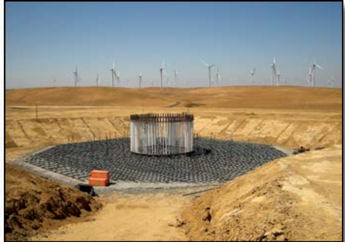
Project: Shilo II Wind Farm Contractor: M.A. Mortenson Co. Location: Rio Vista, CA Photo: enXco & Mortenson Co.
