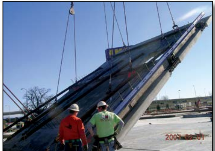
Project: Portland IKEA General Contractor: S D DeaconConcrete / Tilt up Contractor: Whitaker/Ellis Builders Inc. Location: Portland, OR
