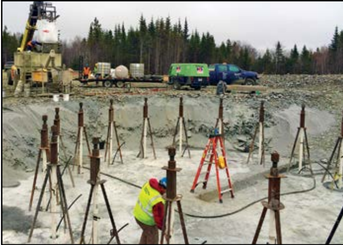
Project: Bingham Wind Project Contractor: Reed & Reed/Maine Drilling & Blasting Designer: Barr Engineering Location: Bingham, ME
