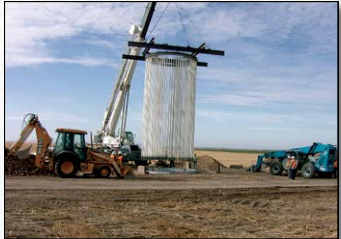
Project: Windy Flats Wind Farm Contractor: Dressel Enterprises, Inc. Location: Goldendale, WA
