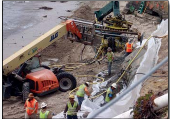
Project: East Cliff Drive Bluff Stabilization Contractor: Drill Tech Drilling & Shoring Location: Santa Cruz, CA
