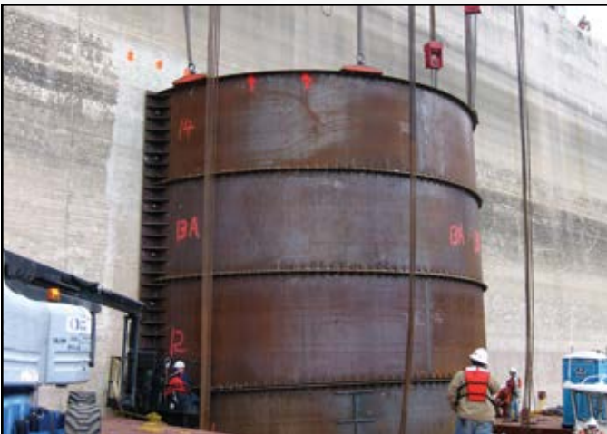
Project: San Vicente Dam Raising Contractor: Barnard Construction Location: San Diego, CA
