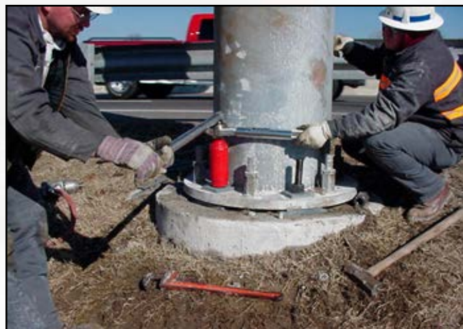
Project: Tennessee DOT Cantilever Sign Retrofit Contractor: Thompson & Thompson Location: Throughout Tennessee
