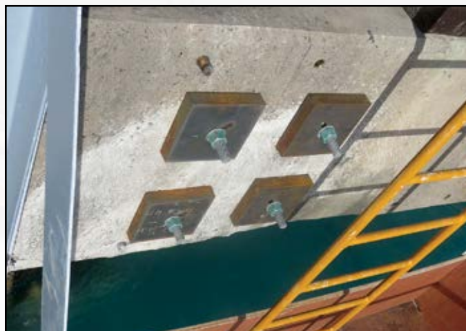
Project Name: Repairs to Deep Draft Wharf, Fac. 4028 Contractor: Black Construction Corporation Location: Diego Garcia, British Indian Ocean Territory
