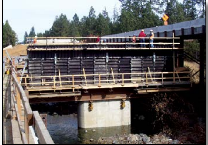
Project: Illinois River Bridge Replacement Contractor: Hamilton Construction Company Location: Cave Junction, OR
