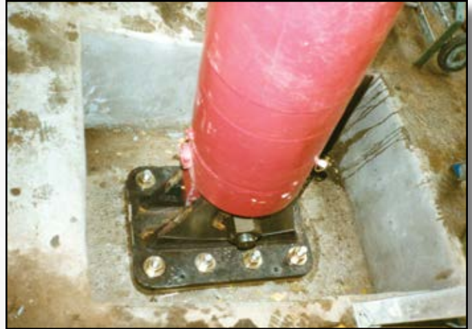
Project: Popp's Ferry Bridge Rehab Contractor: Coastal Marine Contractors Location: Biloxi, MS
