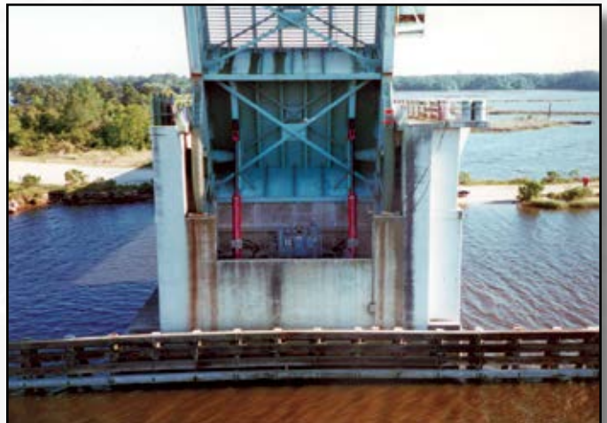
Project: Popp's Ferry Bridge Rehab Contractor: Coastal Marine Contractors Location: Biloxi, MS
