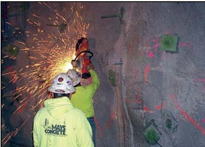
Project: 1-70 Hanging Lake Tunnel Cross Passage Contractor: Mays Constuction Specialties Inc. Location: Glenwood Canyon, CO
