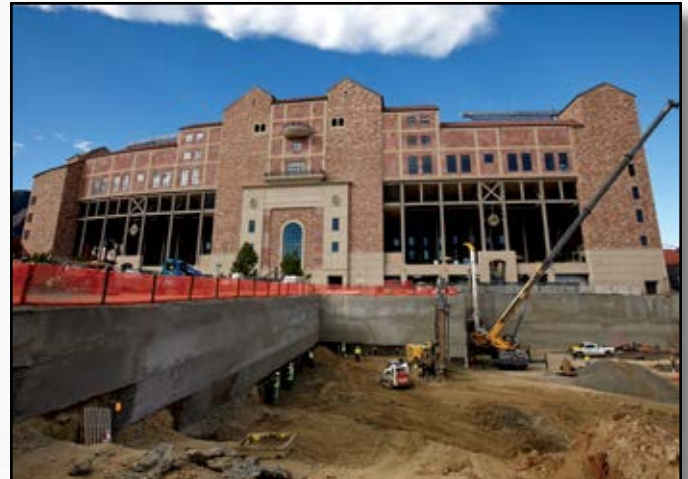
Project: University of Colorado Boulder Athletics Complex Contractor: Nicholson Construction Location: Boulder, CO
