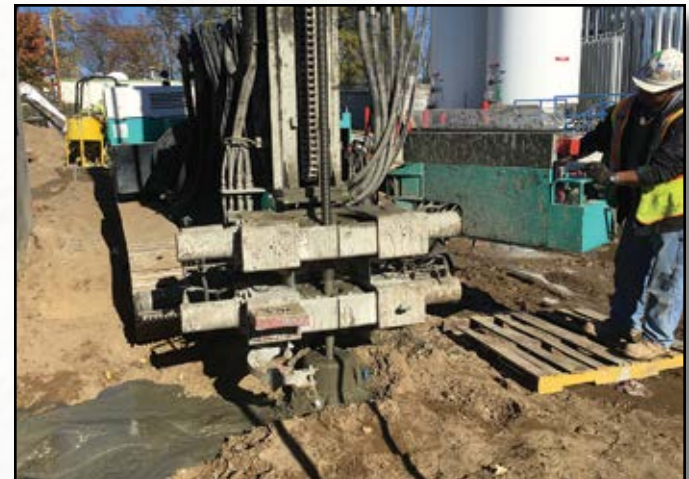
Project: Holland Wastewater Treatment Plant Contractor: Spartan Specialties Location: Holland, MI
