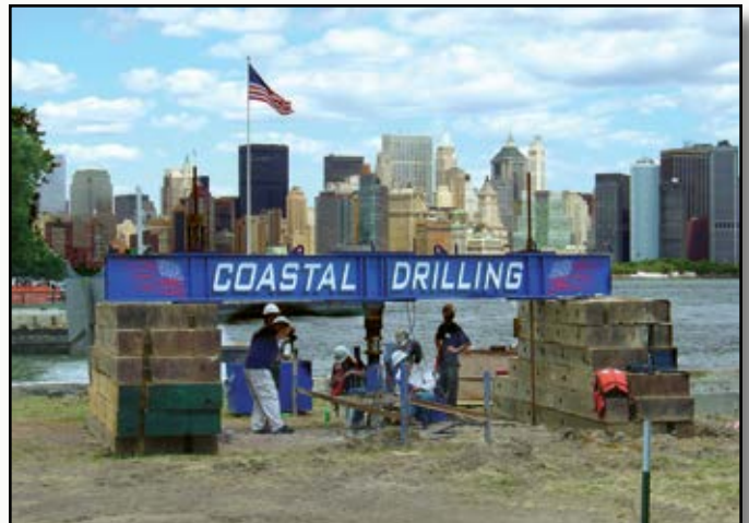
Project: Ellis Island Seawall Rehabilitation Contractor: Coastal Drilling Co. Location: New York, NY
