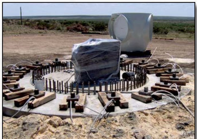
Project: Sand Bluff Wind Turbines Designer: Patrick & Henderson Location: Big Spring, TX
