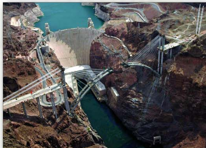
Project: Colorado River Bridge General Contractor: Obayashi / PSM, JV Post-Tensioning Supplier: Schwager Davis, Inc. Location: Hoover Dam, NV
