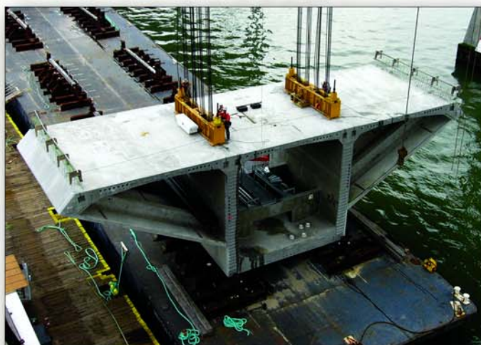
Project Name: San Francisco - Oakland East Bay Skyway Bridge Designer: T.Y. Lin / Moffet & Nichol, JV Contractor: Kiewit / FCI / Manson, JV Post-Tensioning Supplier: Schwager Davis, Inc.
