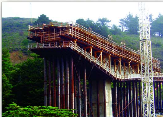
Project: Devil's Slide Bridge Contractor: Disney Construction Post-Tensioning Supplier: Schwager Davis, Inc. Location: Pacifica, CA
