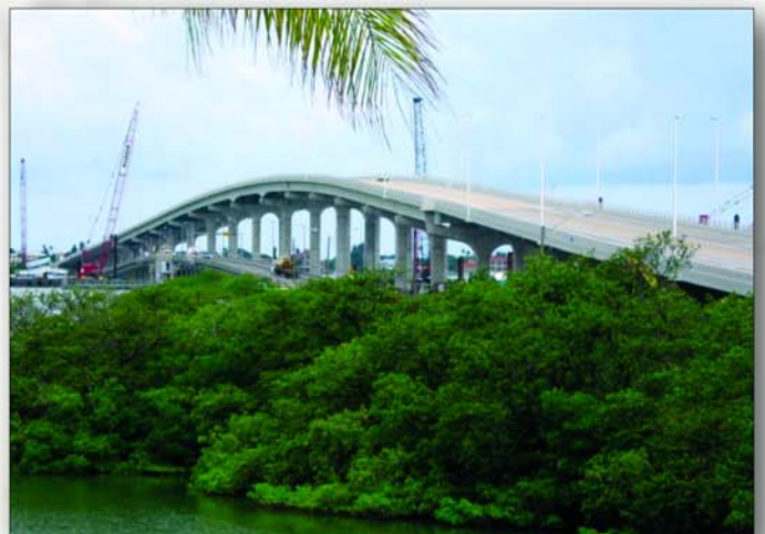
Project: Belleair Beach Causeway Contractor: Johnson Brothers Corporation & Misner Marine Construction / VSL Location: Pinellas County, FL
