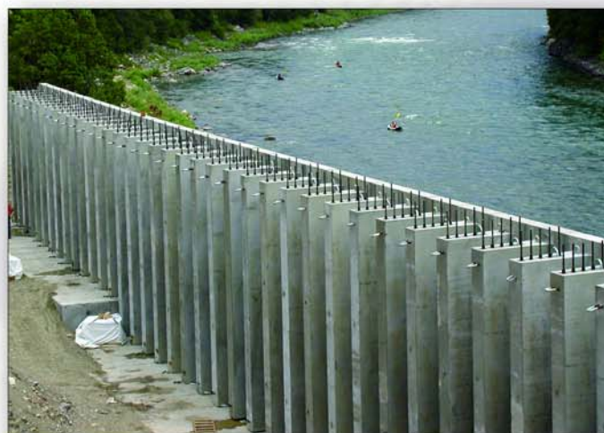
Project: Precast Post-Tensioned Panel Wall Contractor: Morgan & Oswood Location: Hoback Junction, WY
