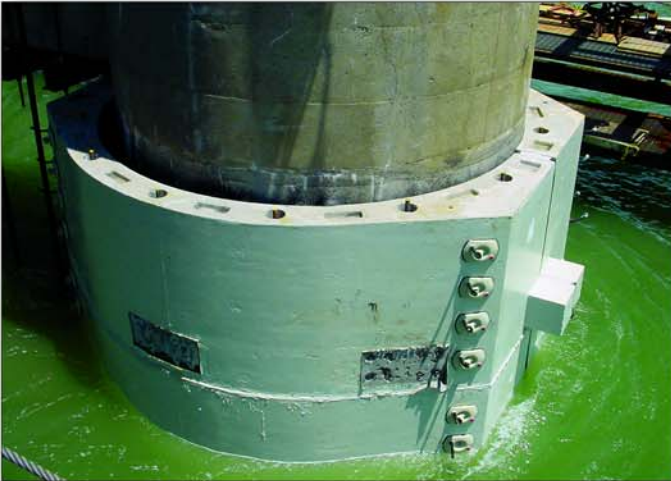
Project: Richmond - San Rafael Bridge Contractor: Tutor Saliba Location: San Rafael, CA
